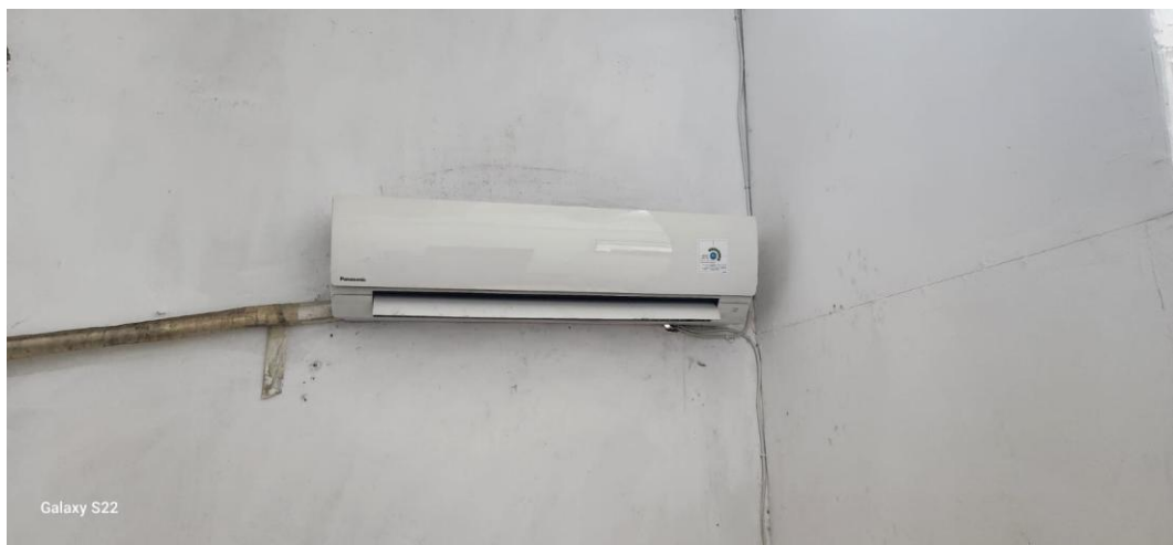
Gambar 1. 13 AC Ruang Server
